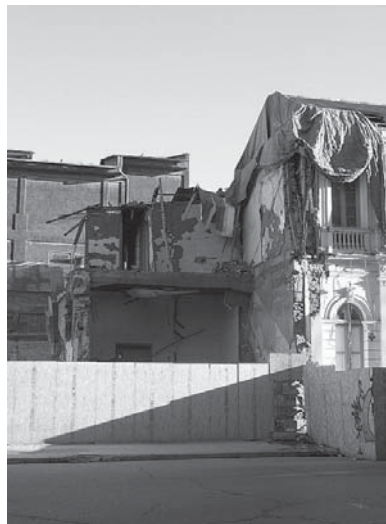
Earthquake damage on main plaza Curico, Chile, February 2010
